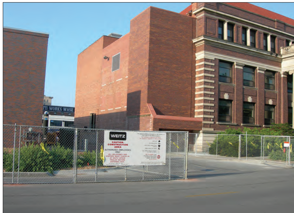
Weitz Construction fenced off the construction area in late June to begin work on the Temple Building renovation.
