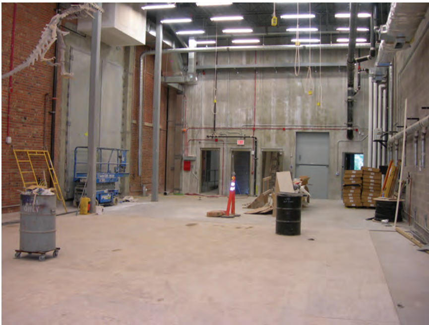
The new scene shop space east of the Howell Theatre on May 23, 2007.
