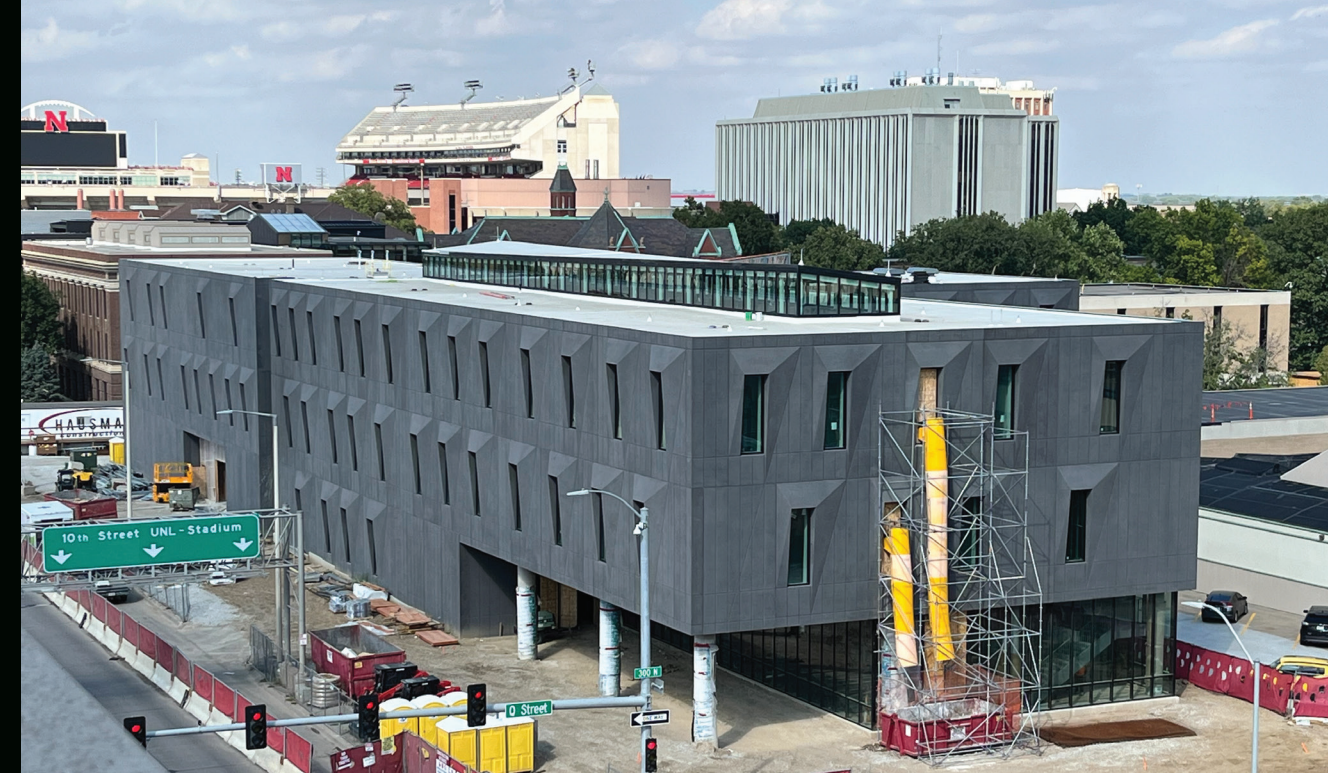
Construction continues on the new music building at 10th and Q streets. This photo is dated Sept. 20, 2024. Photo by Kathe Andersen.
